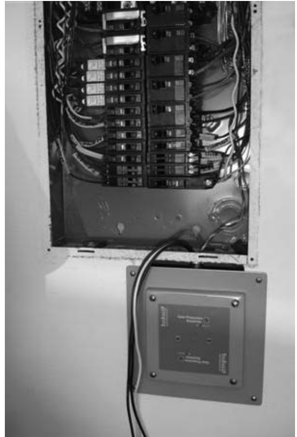
Fig. 5 Sample picture of ground connection to AC panel
