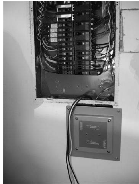
Fig. 8 Sample picture of ground connection to AC panel
