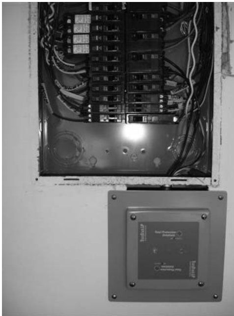
Fig. 9 Sample picture of unit installed and Operating properly
